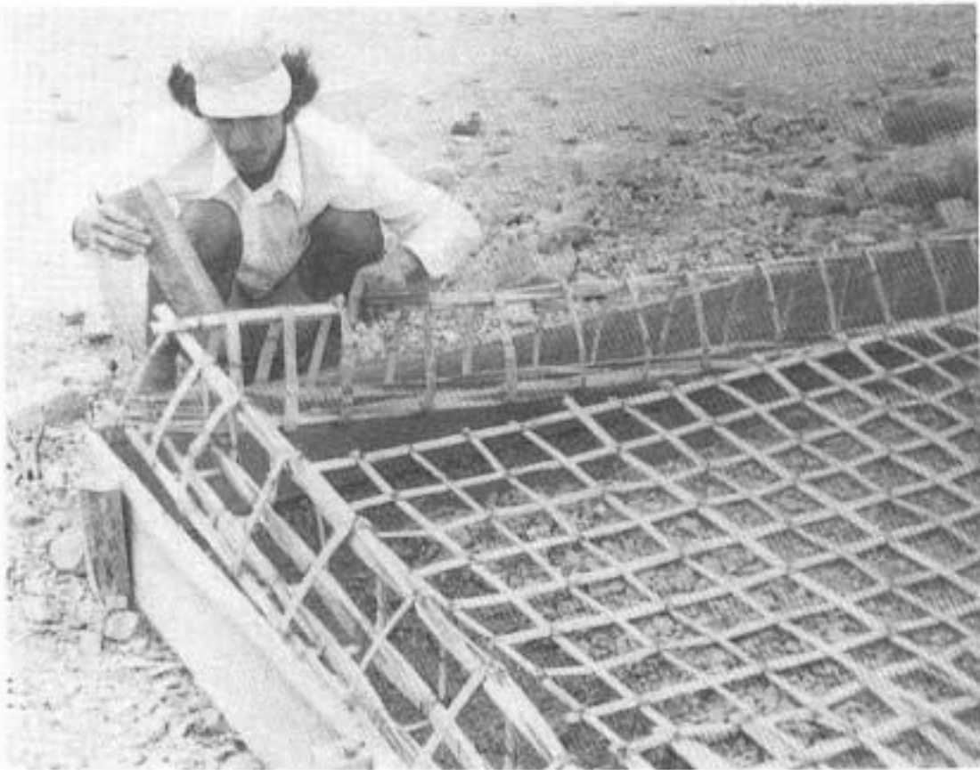
Fig. 12: Peripheral beams of the slab foundation were reinforced with bamboo cables, with satisfactory results
