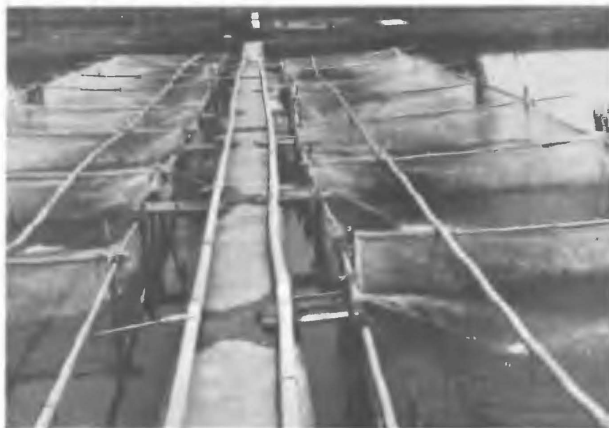
Fig. 20. Net cages set along the concrete bank wall and the piping system for water supply.
